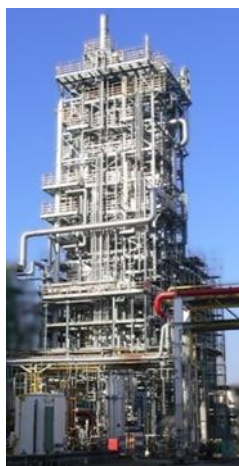
Figure 2. Overview of the Test Furnace
